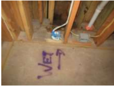
Wet area in fourth level from roof leakage
