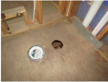
Hole in sub floor in second level toilet closet
