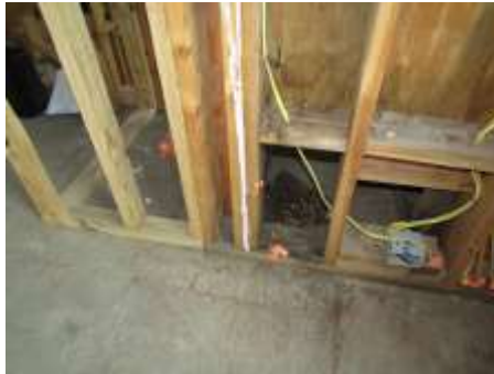
Water in second level south floor
