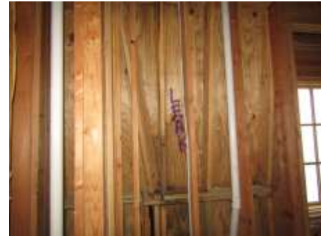
Active roof leakage in fourth level
