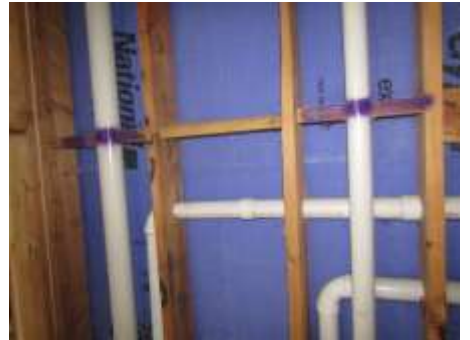
Missing strap on PVC drain pipes
