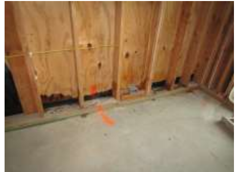
Water at base of common north wall from Unit #35
