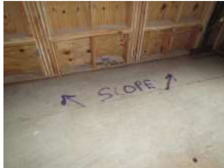
Floor deflections in second level kitchen
