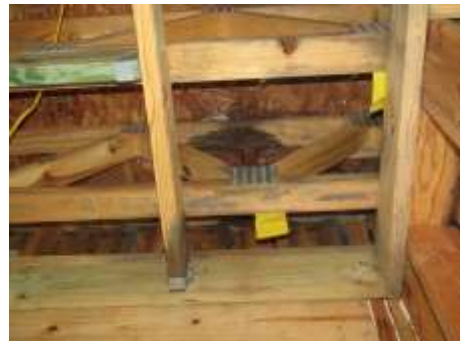
Stained second level sub floor from previous leaks
