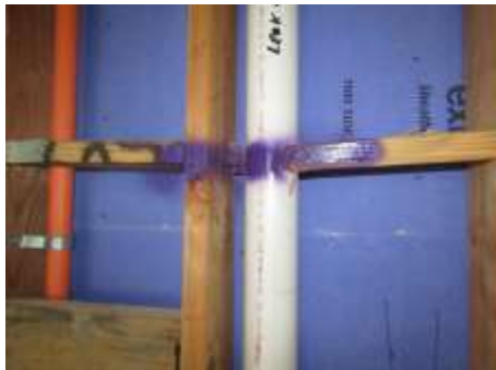
Missing strap on second level PVC drain pipe
