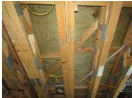
Infrared revealing moisture from water on fourth level balcony deck
