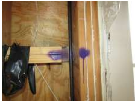
Missing strap on gas pipe
