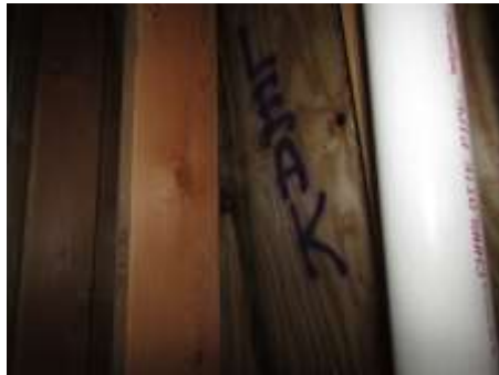
Leak in fourth level from roof
