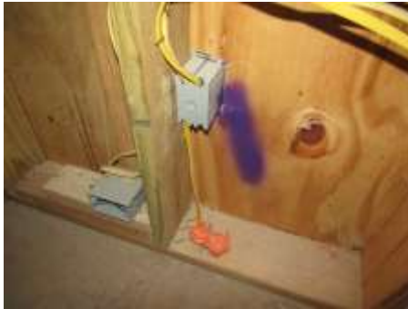
No fire stop sealant at outlet to balcony
