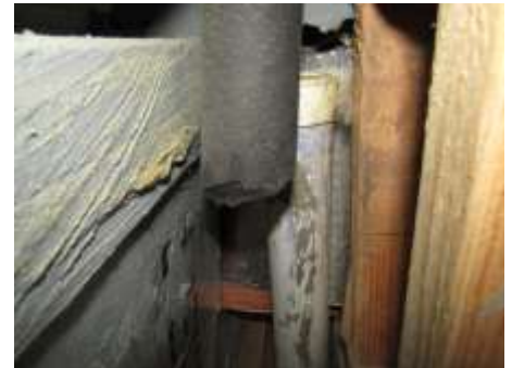
HVAC primary drain not installed
