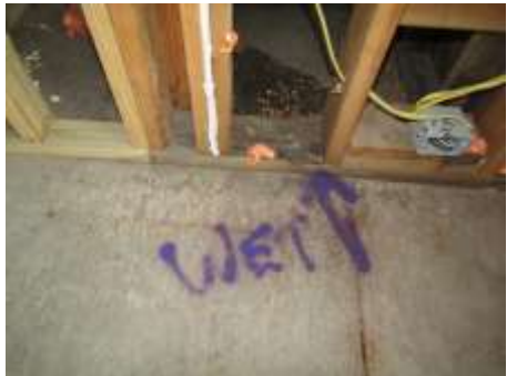
Wet sub floor in second level
