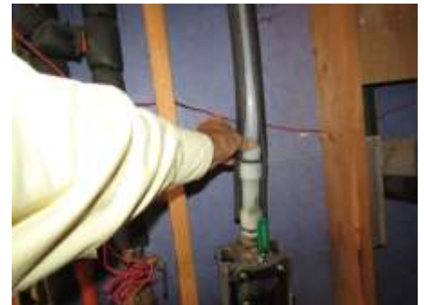
Loose Pex water line piping in garage
