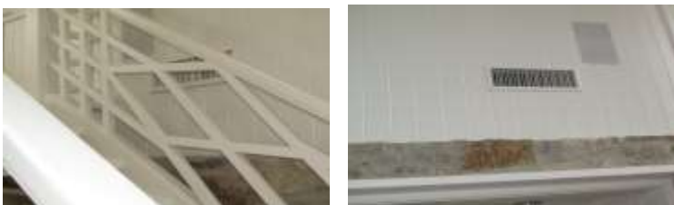
No air supply from one of two south lower family room registers
