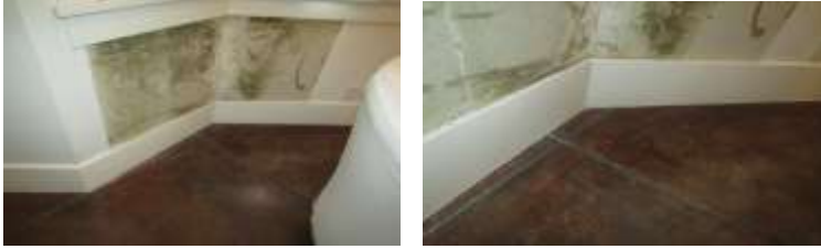
Mold propagation on drywall under 1 st southeast bedroom window
