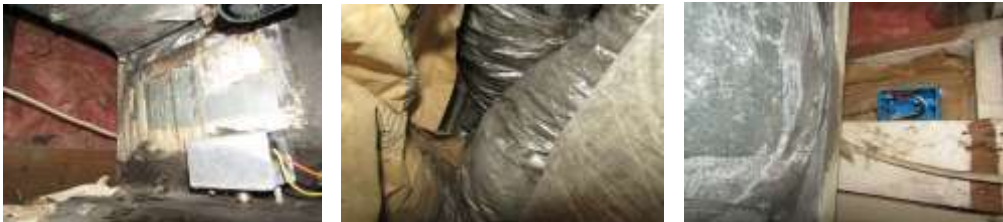
Black organic matter on 2 nd level HVAC ducts and plenums...missing cover on jbox
