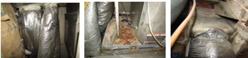
Black organic matter on 2 nd level south HVAC ducts and equipment
