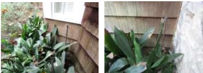
Sprinklers close to exterior building
