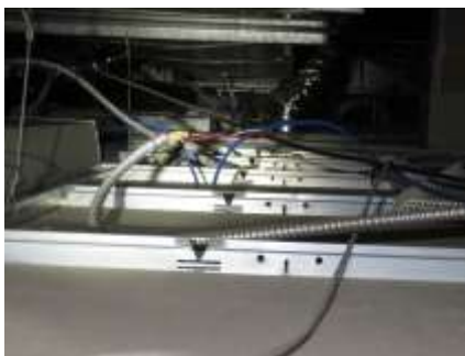
Cut and exposed wires above west ceiling
