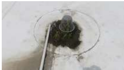
A/C drain not installed into roof drain
