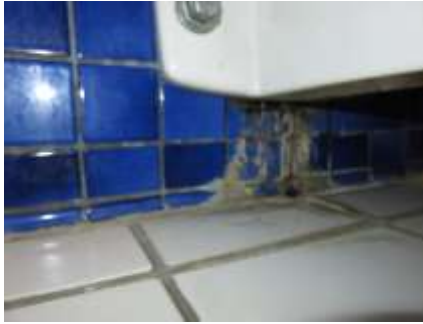
Stains and leakage off toilets
