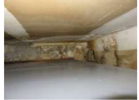
Sheetrock wall damages and mold
