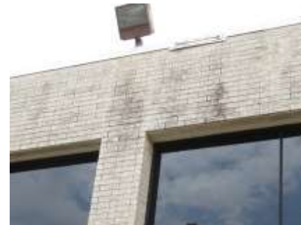
Stained brick off roof scuppers
