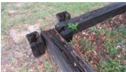
Damaged wood railroad ties
