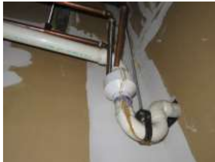
PVC trap with previous leaks in elevator equipment closet
