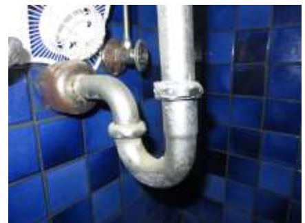
Corrosion on P trap
