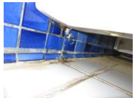
Leakages of toilet
