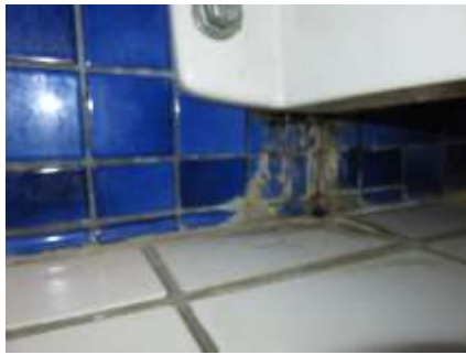
Stains and leakage off toilets
