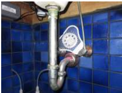
Corrosion on chrome P traps at all lavatories
