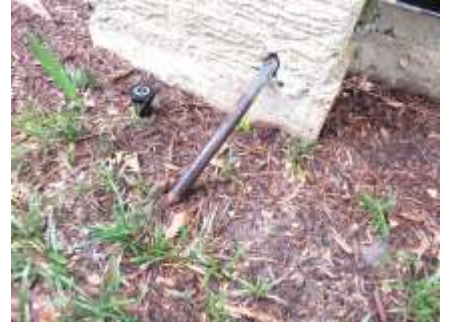
Rusted conduit at east exterior
