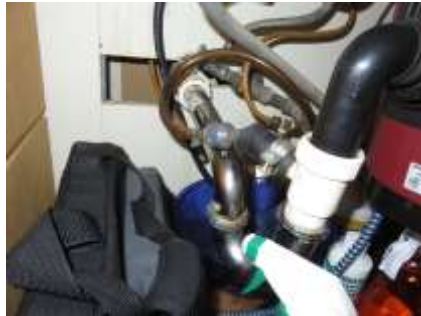
Poor dishwasher drain connection in upper east kitchen
