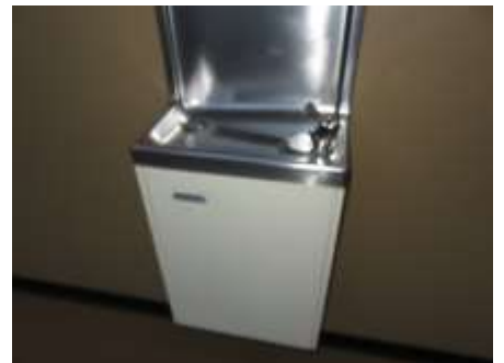
Water cooler not operative
