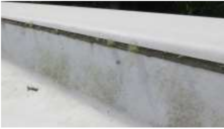
Plant growth along southeast roof
