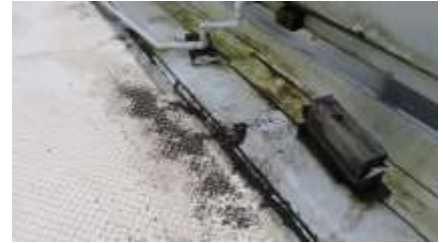
Stains and debris off HVAC on roof
