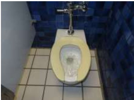
Weak flush on all toilets
