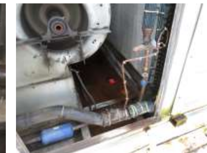
Rust and water in Trane HVAC
