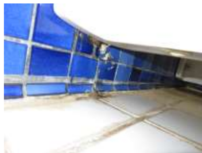
Leakages off toilet
