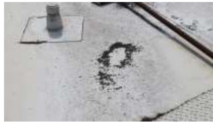
Debris on roof from ponding water
