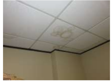
First level east kitchen acoustic tile stains
