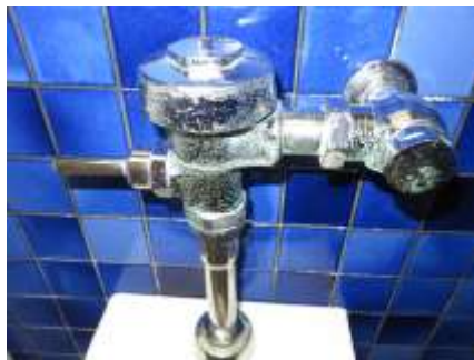
Corrosion on men's urinal fixture
