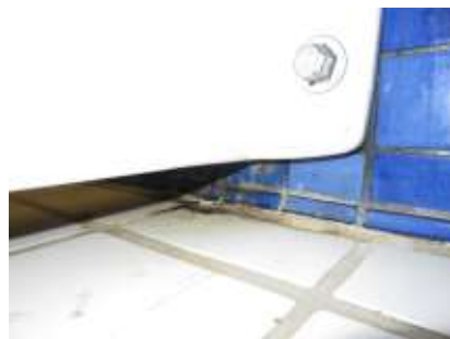
Leaks off toilets
