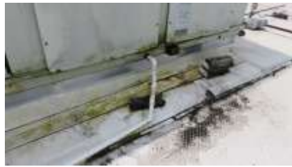
Excess stains and water off HVAC equipment on roof
