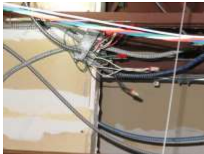
Exposed wires above ceiling tiles
