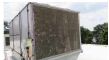
Hail damage to Carrier coil
