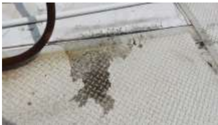
Water under mat around HVAC units
