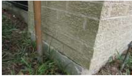
No weep holes at base of brick columns
