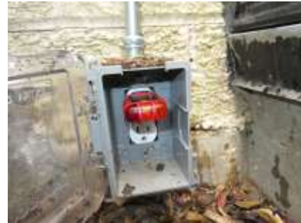
No power on exterior north outlet
