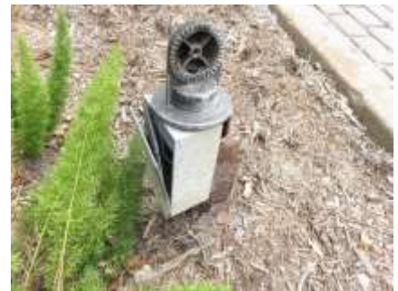
Broken junction box at front exterior sign
