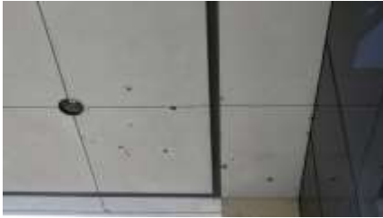
Stains and mud wasps on stucco ceiling at front exterior
