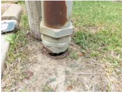
Rusted metal conduit for main feed into building
