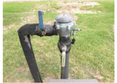
Sprinkler PVB valve on off mode
