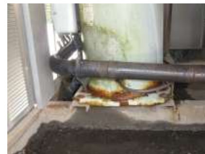
Rusted compressor on Trane unit
