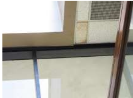
Stained acoustic tile off skylight
