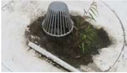
Debris and vegetation at roof drain from HVAC drain
