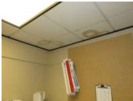
Stained tiles in upper west storage closet
