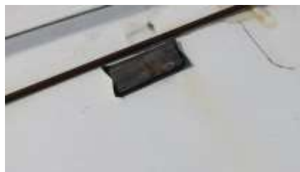
Loose 2x4 supporting conduit
