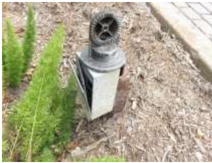
Broken junction box at front exterior sign
