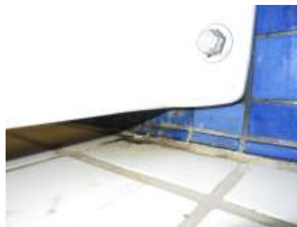
Leaks off toilets
