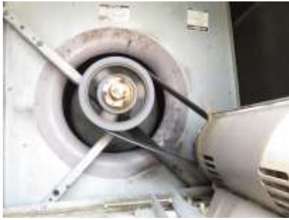
Mold/mildew on Carrier unit air handler and loose belt
