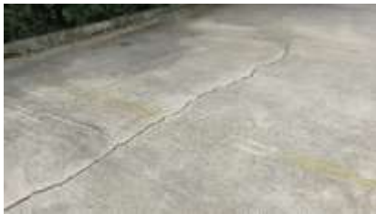
Fractures in south parking lot concrete
