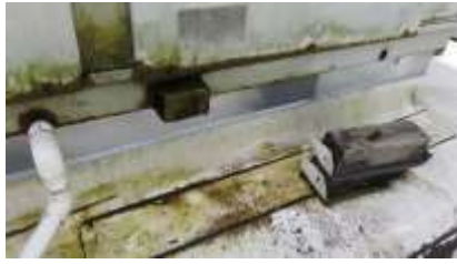
Excess rust and water leakage off Trane unit
