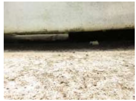
Debris at south drain scupper
