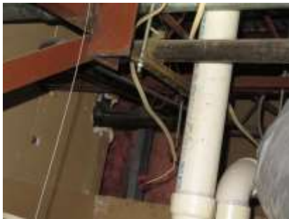
Exposed cable wires
