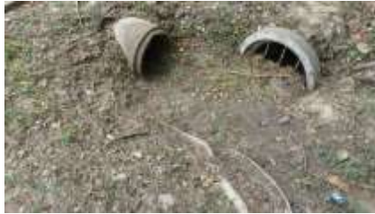
Debris and clogged drain culvert and pipes
