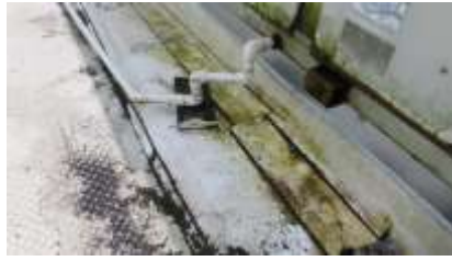
Missing trap off Trane HVAC unit drain pipe
