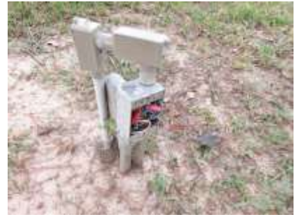
Missing cover on exterior east junction box
