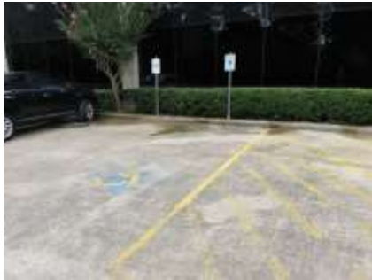
Poor marking for handicap parking
