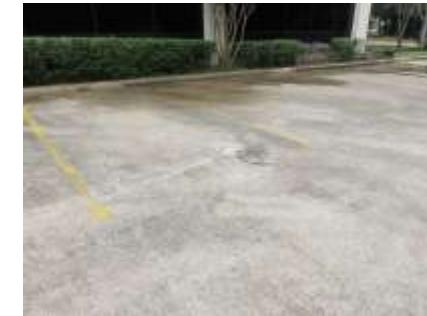
Poor marking for parking
