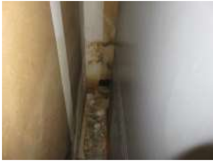
Sheetrock damages and mold
