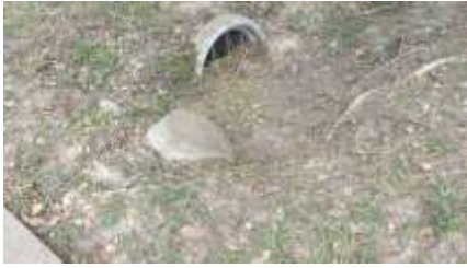
Clogged drain in culvert
