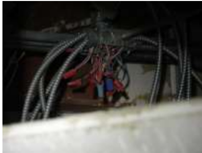
Exposed and unused cable wire above first level men's bathroom
