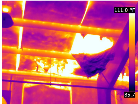
Images of heat on insulation from compromised insulation
