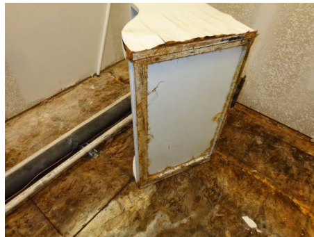
Stained floor and cabinet in second level equipment room
