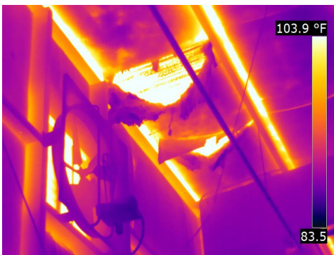
Image of torn insulation under roof
