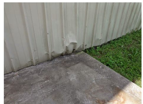
Damaged lower siding
