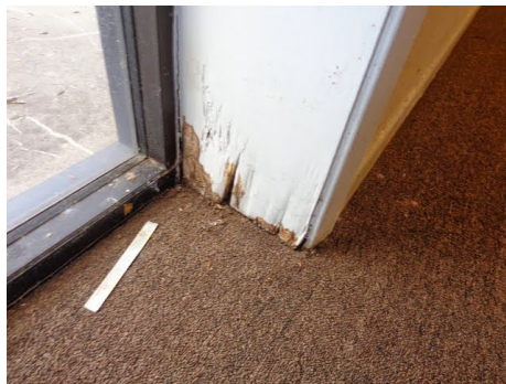
Damages inside office
