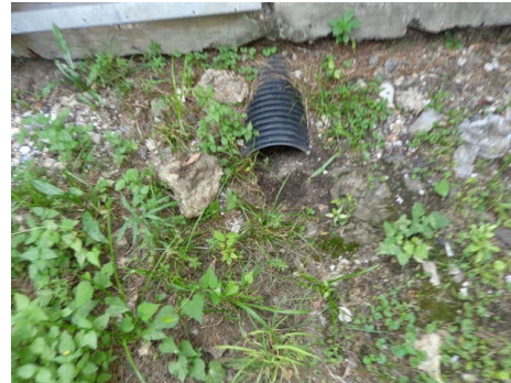
Clogged drain at west side
