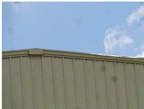
Damaged upper north edge of roof
