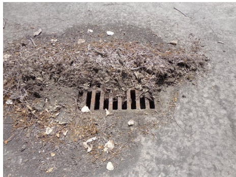
Clogged east drain in parking lot
