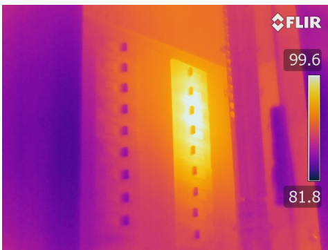
Heat on interior breaker panel breakers during operation of equipment
