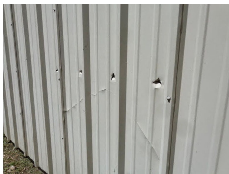
Holes in siding
