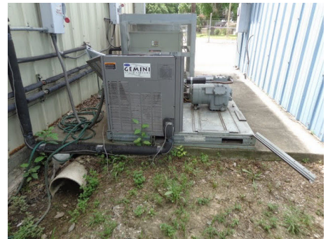
Both large A/C units vandalized
