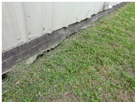
Erosion at northeast area
