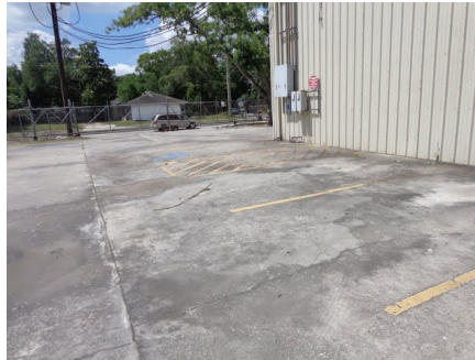
Worn paint markings for parking
