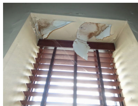
Damages inside office window
