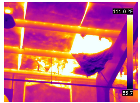
Torn and damaged insulation under roof
