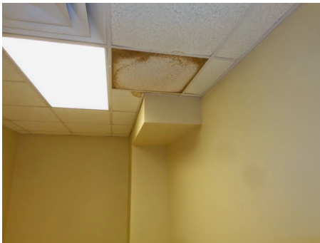
Ceiling tile damages
