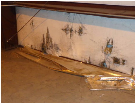
Stained and damaged interior wall insulation
