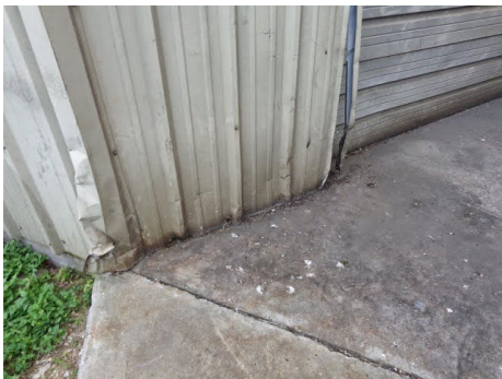
Damaged exterior siding and trim
