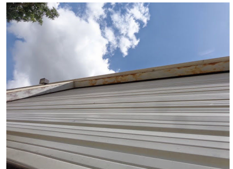
Rusted trim on bay doors
