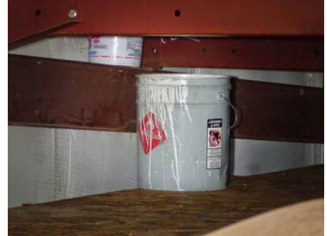
Buckets in attic
